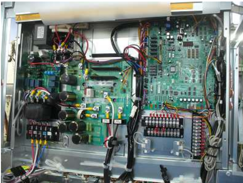
Air to water unit
