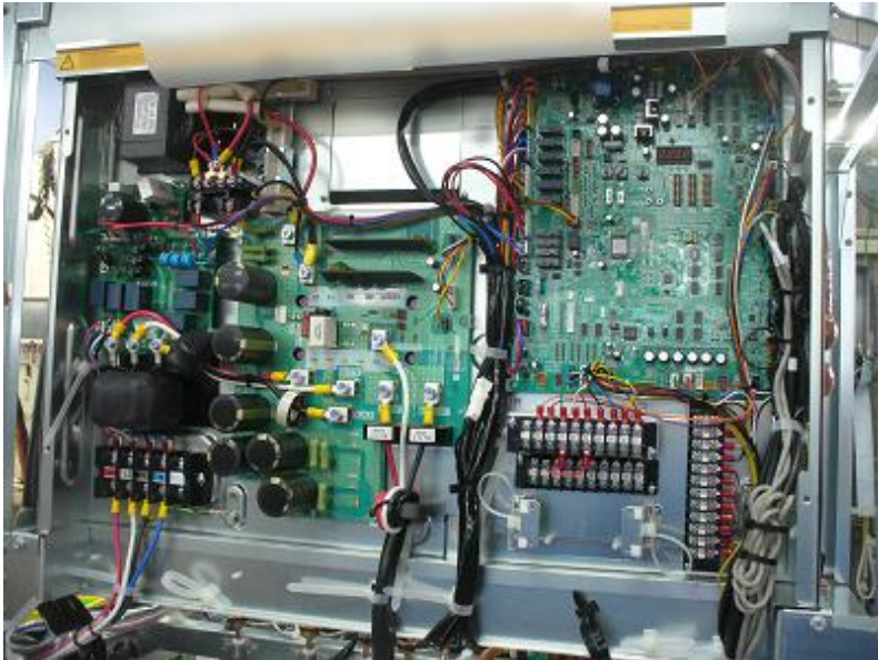
Air to water unit
